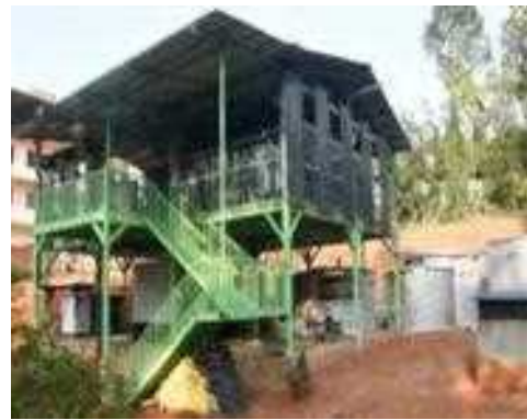
1 MLD STP at Kozhikode medical College
