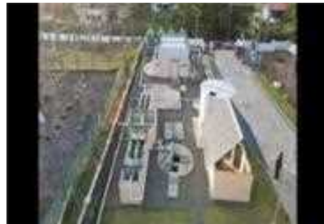
1 MLD CSTP at Padanappalam, Kannur
